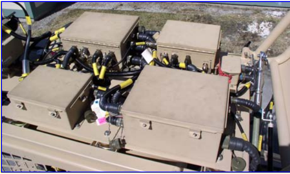
Figure 3. Platform Control Components (PCC) on Roof-Rack
